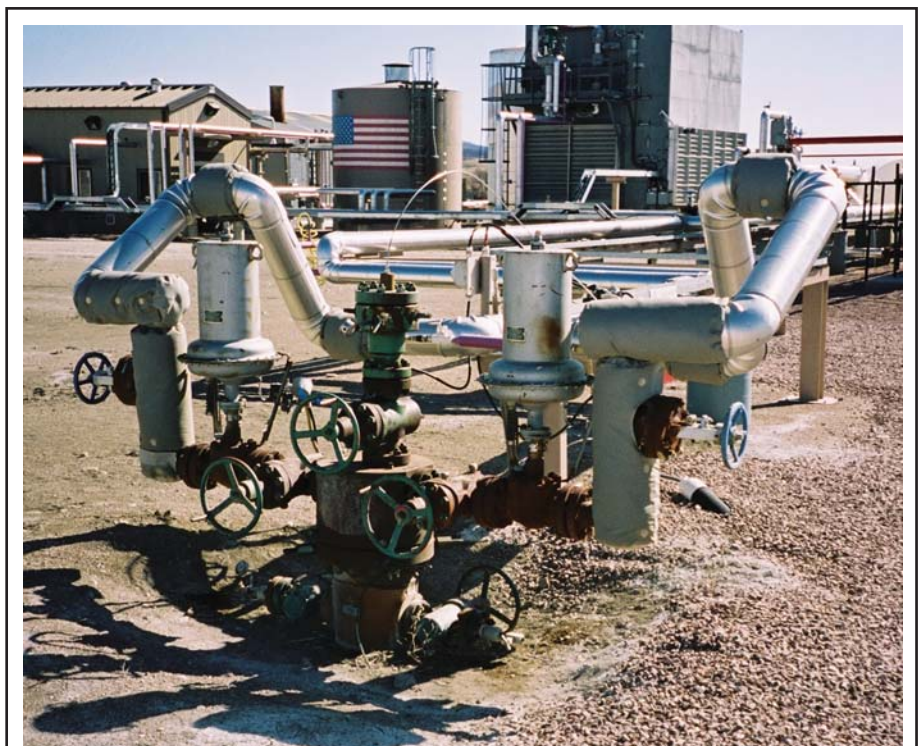
Improving production and recovery rates from the LAK Ranch Field requires the right technologies, a bit of experimentation and healthy commodity prices. Longer term, part of the revenues from the EOR operations may be used to explore the potential of deeper horizons underlying the field that were identified in new 3-D seismic data acquired over the area last year.
