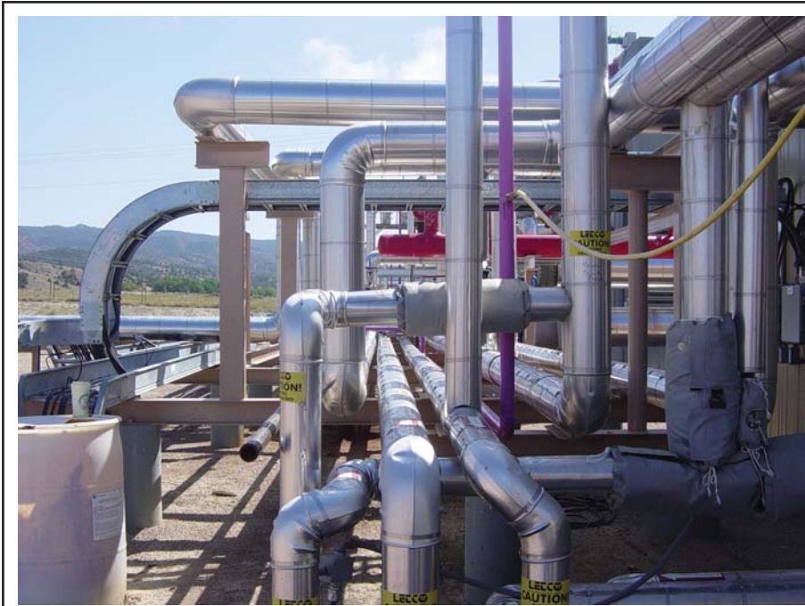
The surface facilities at LAK Ranch include a computerized control center, steam generator, aerial cooler, heater treater, oil production and storage equipment, and a water separation unit to treat and reclaim steam and co-produced water. The day-to-day operations of the project are monitored and controlled using state-of-the-art automation systems.
