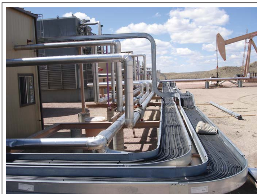
The LAK Ranch steam plant includes a 27 million Btu generator capable of moving more than 700 barrels of oil a day. The plant is highly automated so that it requires only minimal staff.
